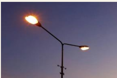
Installed 75 streetlights in Susan's Bay to be powered by the biogas plant
